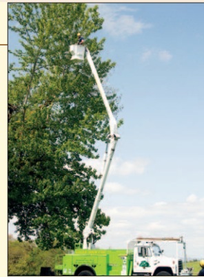
Due to the history of large branch failure the cuts were done from the safety of a bucket truck
